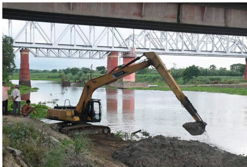
FIGURE 6 | Post-construction removal of soil and debris from the river bed and banks by NHA. (Curtsey: The Telegraph Online, 02.07.2024).
